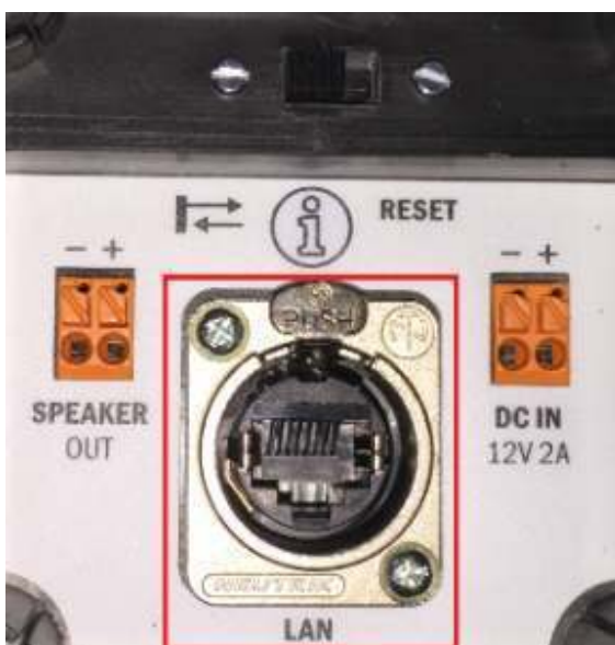
Figure: LAN Connection
